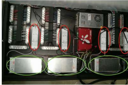
Figure 12: Light-box electronic housing. The components marked with red are the LED dimmers while the components marked in green are the HRP 600 power supply units.
